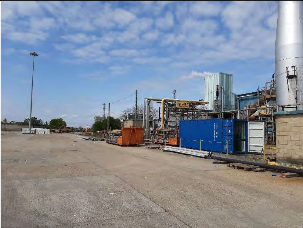
2. Boiler House Looking NW showing staining at base of blockwork wall.
