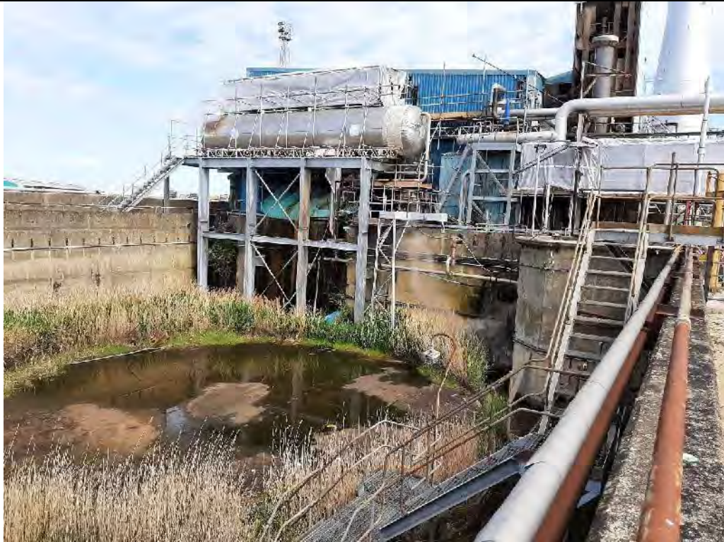
3. Boiler House Looking E showing one of the former sunken storage tank bases (former gas oil for the boiler house). The boiler house is now fired by natural gas.
