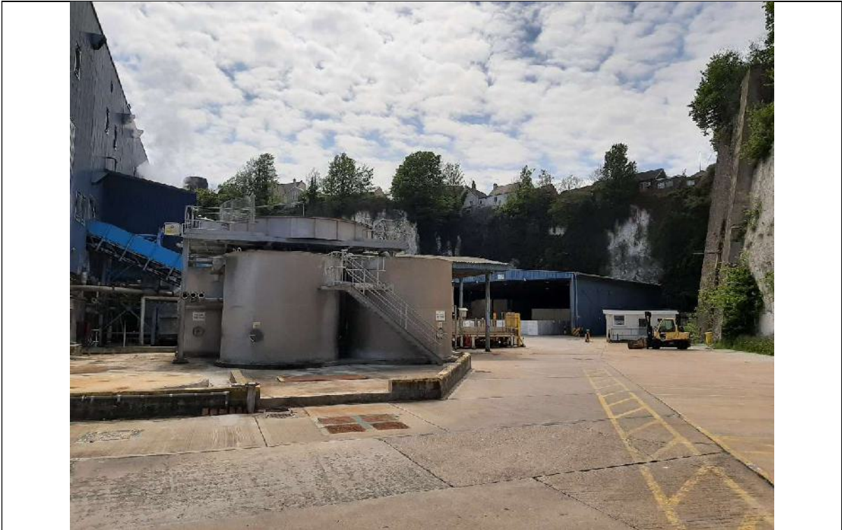
7. Storage tanks in southern area looking SE.
